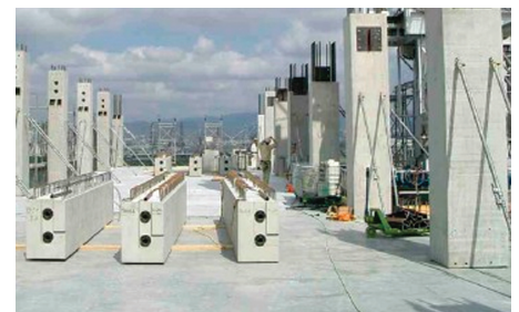
Photo 17 プレキャスト工法の施工例 An example of construction using a precast concrete method
