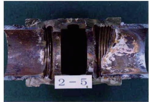
Photo 2 給水用硬質塩化ビニルライニング鋼管の異種金属接触腐食 (32A, 6年, ライニング材剥離後) 1) Galvanic corrosion of rigid polyvinyl chloride lining steel pipe for water supply (32A, and 6 years, after taking off lining material)
