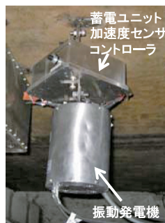
Photo 5 振動発電機設置状況 Vibration energy harvester
