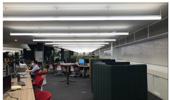
Photo 21 Workspace with pendant illumination fixture
