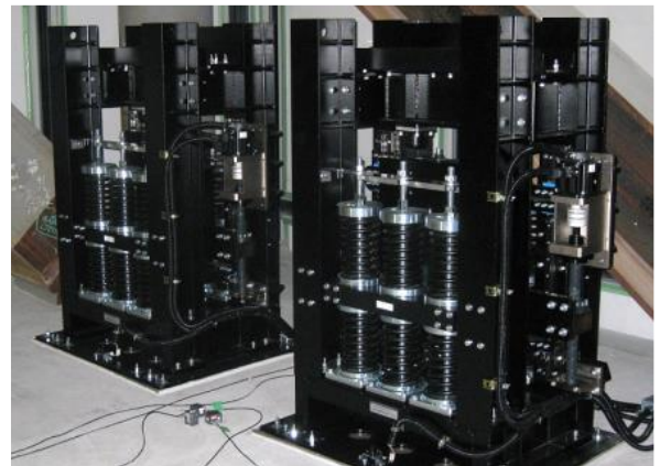
Photo 4 Example of HMD installed in the building on the receiving side
